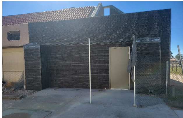
Fire Damage Repair, Bay Ave. Photos by Grand Jury
